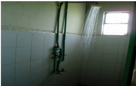
Hot water in dorm bathrooms heated by solar panels on roof
